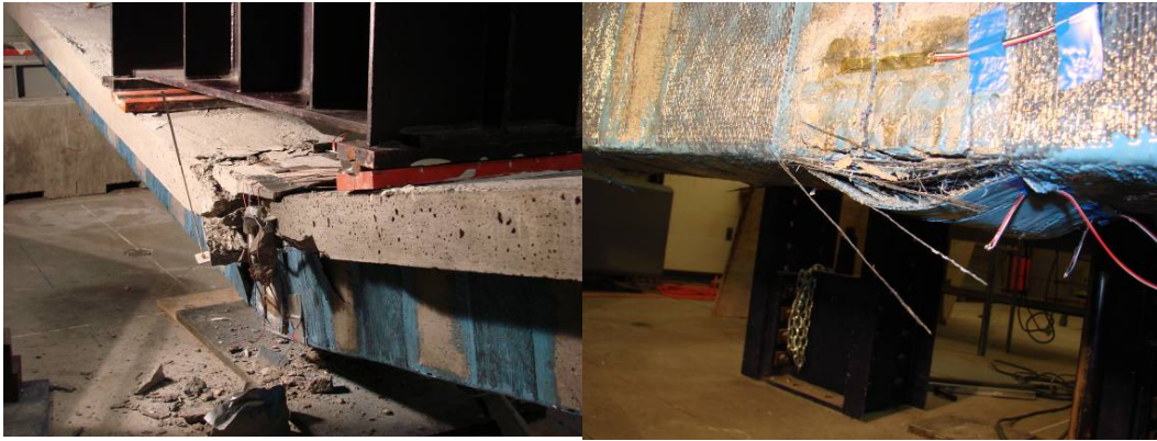
Figure 1: Failure of beam T3 by FRP rupture.
